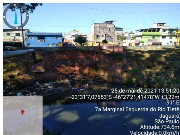
Figure 38. Site #3 – Just after gabions have taken failure
