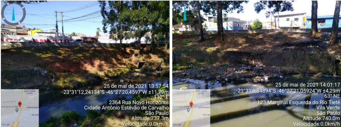
Figure 39. Site #4 – Just after gabions have taken failure
