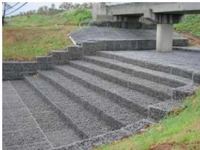
Figure 16. Gabion was used for river cladding under a bridge. Source: Maccaferri (2020).
