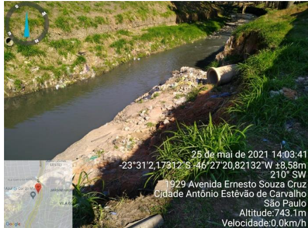
Figure 36. Site #1 – Just after gabions have taken failure
