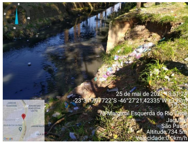
Figure 37. Site #2 – Just after gabions have taken failure
